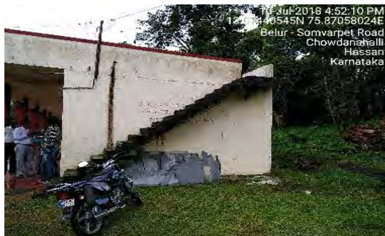
MR Aided High school, Sakaleshpura-Staircase without railings
