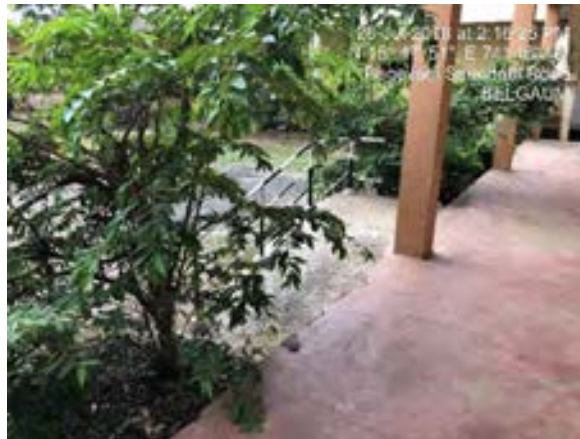
Ramp without double railings and non-accessible through wheel chair Government High School, Belagavi
